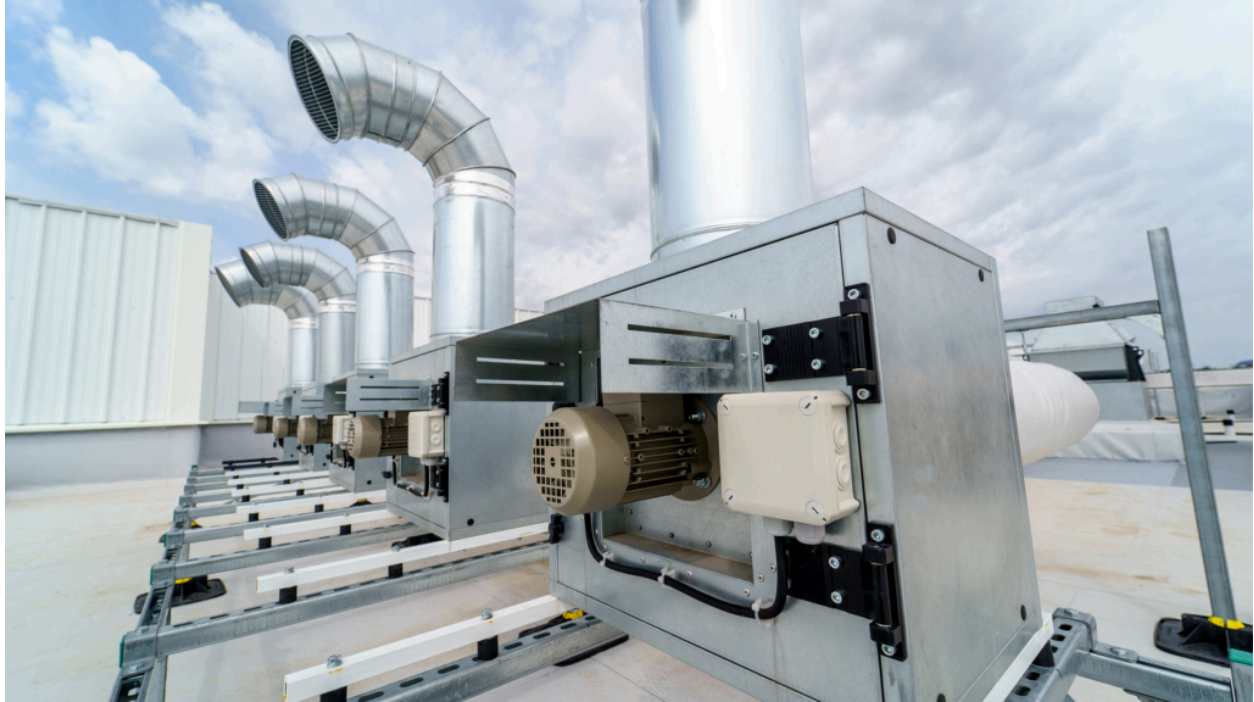
VAV HVAC duct system with pressure sensors and VFD controller
